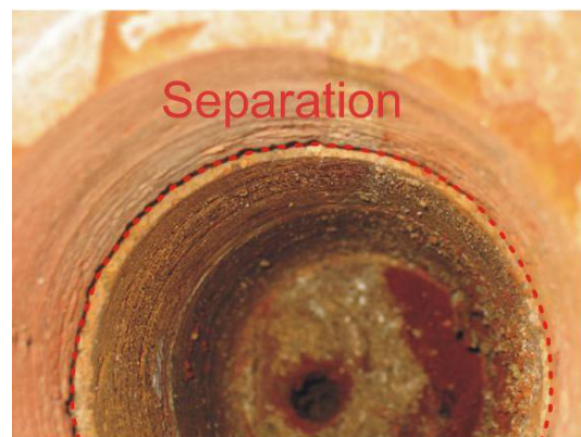
(b) view through core hole showing separation of bottom layer of brickwork
